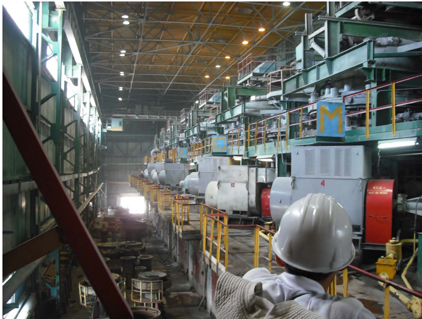
Figure 3: Inside the mineral processing factory of Erdenet.
